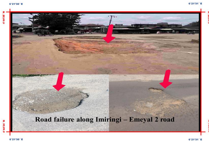
Figure 3: Image of failed portion of Imiringi – Emeyal 2 road
