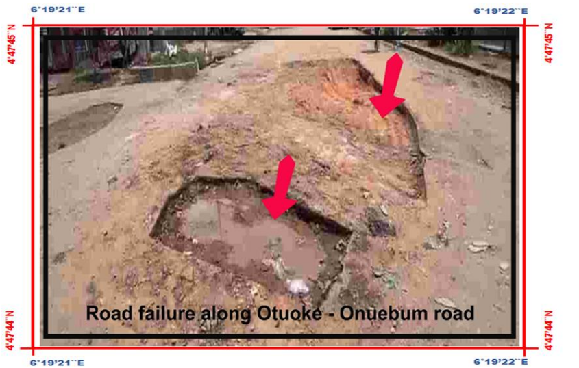
Figure 2: Image of failed portion of Otuoke – Onuebum road.
