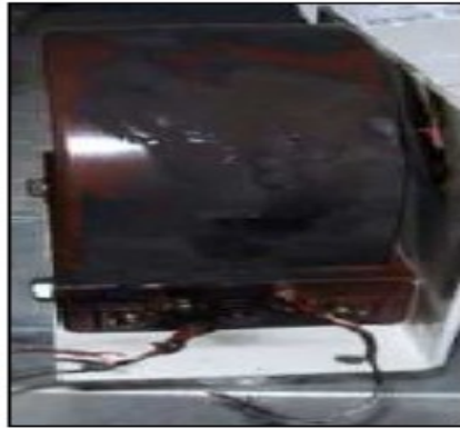
Fig3. Burnt Damping Reactor (ZD) of A-phase for #2 Bus VT
