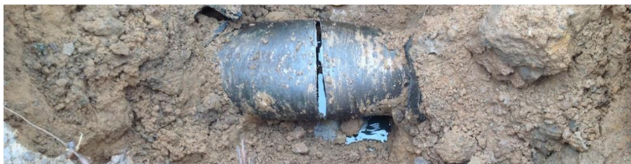
Figure 7: Pipeline sabotage. (Source: author, 2020))
