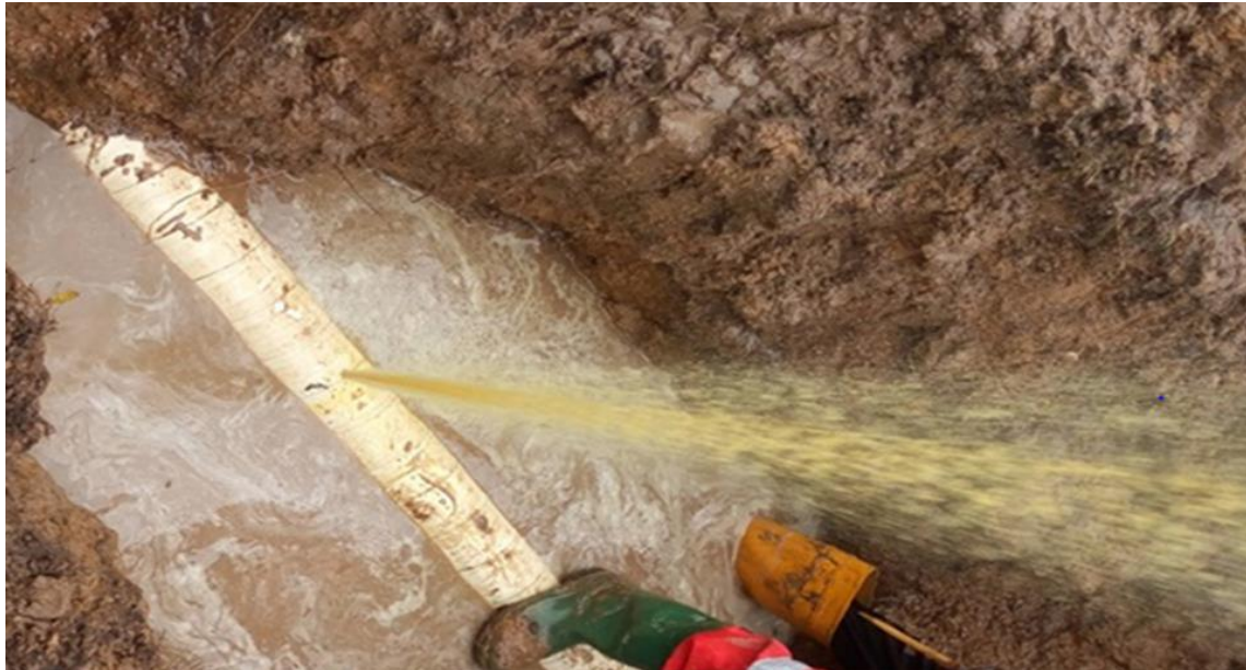
Figure 1: Vandalized pipeline (Source: author (2020))
