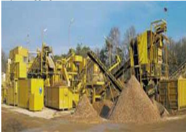
Photo1:Aggregate crushing plant
