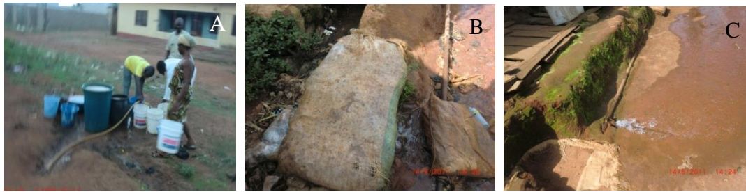
Figure 10: (A) Improper connection at Wukari GRA, (B) Leakage covered garbage sacks at Gembu Kaka Qtrs, (C) Leakage along network at Gembu Mansur Qtrs.
