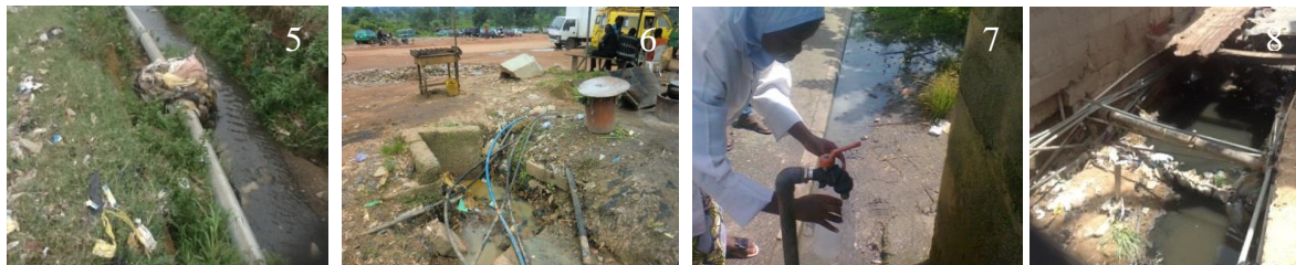
Figures 5 – 8: Pipe connection through insanitary gutter of some pipe borne water supplies
