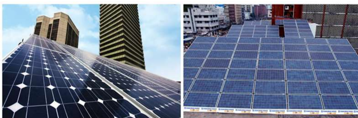
Fig. 6 Rooftop solar at Bangladesh bank(left) , rooftop solar at WapdaBhaban(right) [67]
