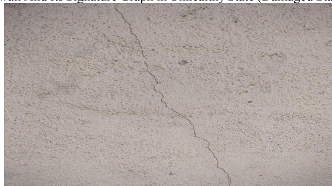
Fig.No.4.7 Load bearing wall (Damaged State)
