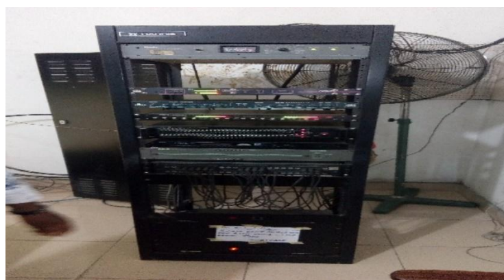
Figure 3: Radio Rivers Studio – Transmitter – link (STL) Equipment
