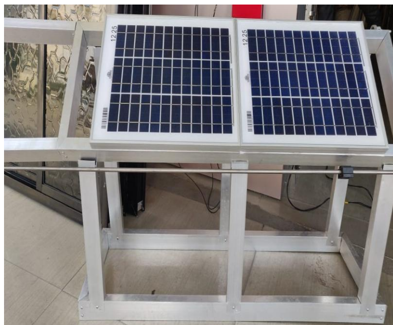
Fig.2: PV panels fixed on the frame
