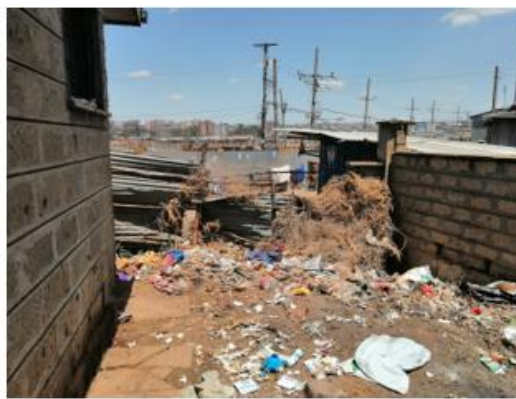
PLATE 9: The collapsed section of perimeter wall Source of plates 8 & 9: Field data, 2023
