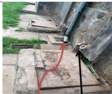
PLATE 12: Rain water and sewage pipes
